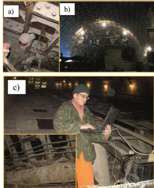
Figure 8. Drilling of a borehole through a cementing port in the segment (a), injections from the trolley-based rig (b), impact echo tests for quality control of injections behind the lining (c).
