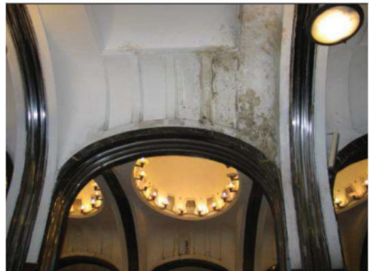
Figure 3. Regular multiple leakages caused deterioration of station finishing.
