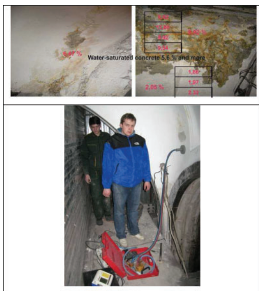
Figure 5. High permeability of concrete caused leakages and structural deterioration.
